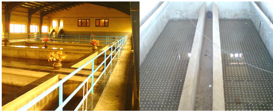
Fig. 5. The view of filtration hall and sand filter bed
