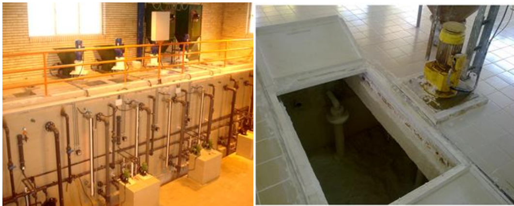
Fig. 3. The view of chemical preparation and injection unit
