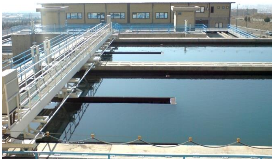
Fig. 4. The view of preliminary sedimentation pool
